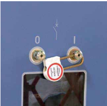
Fig. 10.10 Manual switching ON of circuit-breaker locked by padlock
