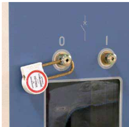
Fig. 10.11 Manual switching OFF of circuit-breaker locked by padlock
