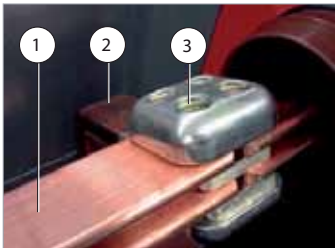
Fig. 5.14 Busbar fastening in a center panel (example shown: PIX 17/24)
