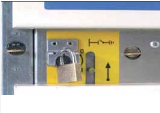
Fig. 10.9 Mechanical lock-out of earthing switch via padlock
